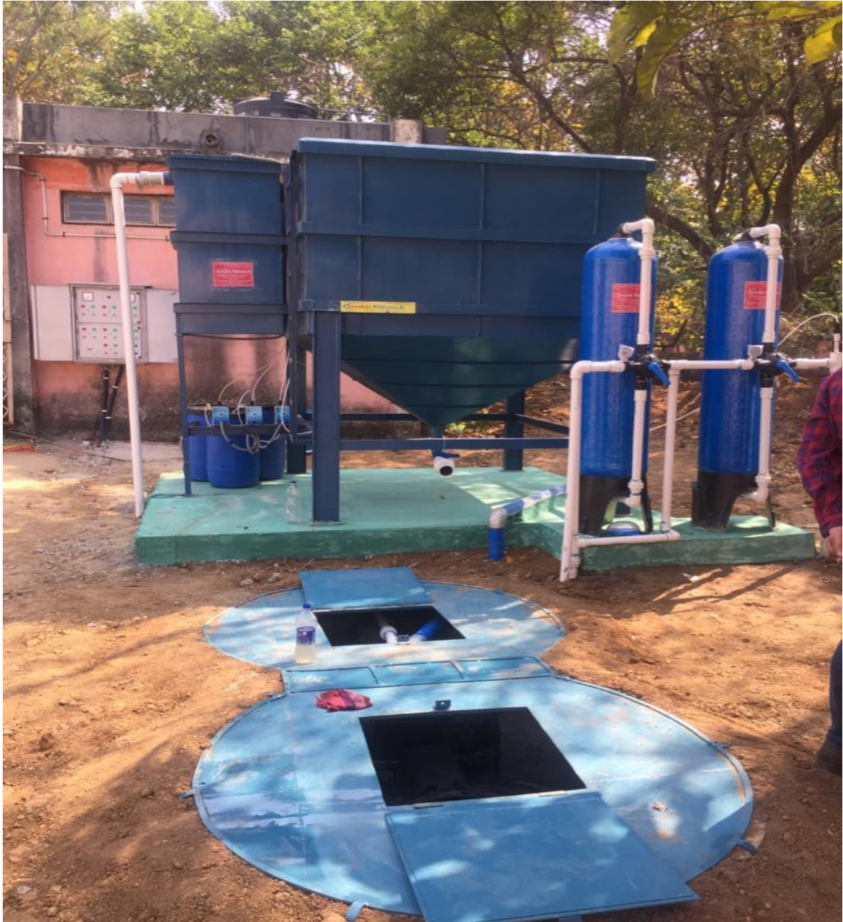
Fig 1: ETP installed at Sapphire Hostel
