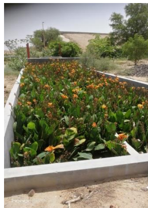
Fig. Decentralised Waste Treatment Plant Bed filter
