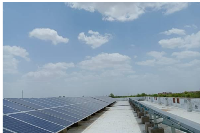
Fig. Rooftop Solar Panels
